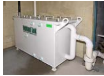
Elevator Sump Pump Interceptors
