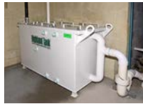
Elevator Sump Pump Interceptors
